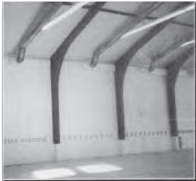
Figure 3.0 Solar Heat Air Duct (Alliance Church)
