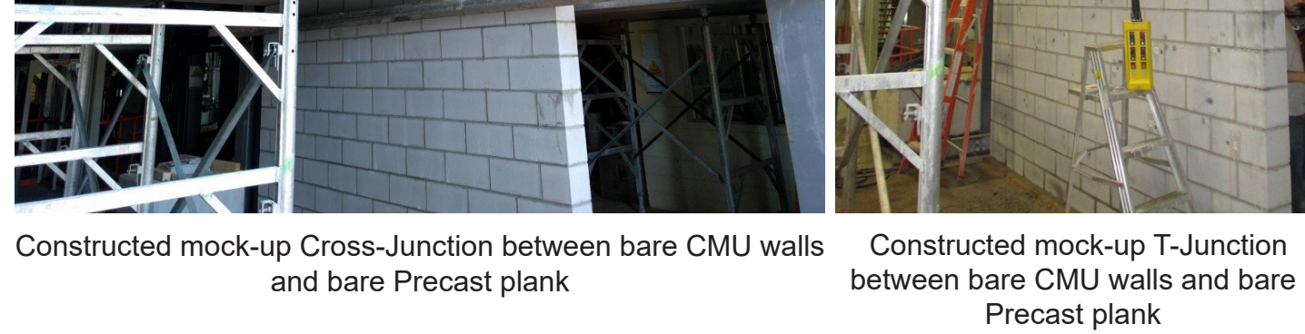
Illustration of the mock-up Cross-Junction between bare CMU walls and bare Precast plank
